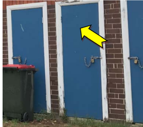
Photo 2. Exterior, throughout, doors - suspected lead-containing blue upper paint system.
