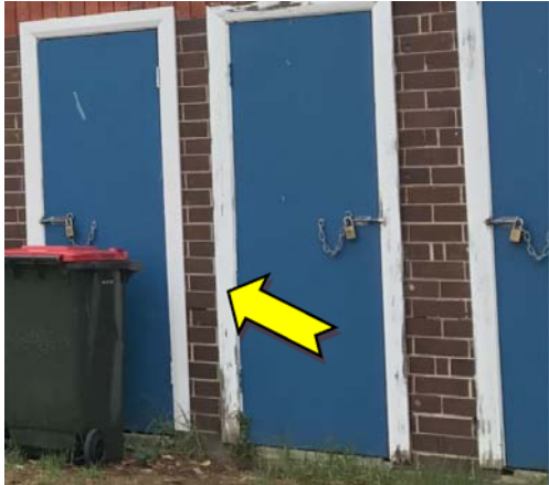
Photo 1. Exterior, throughout, door frames - suspected lead-containing white upper paint system.
